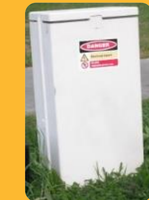
Distribution cabinet (commercial supplies only)
